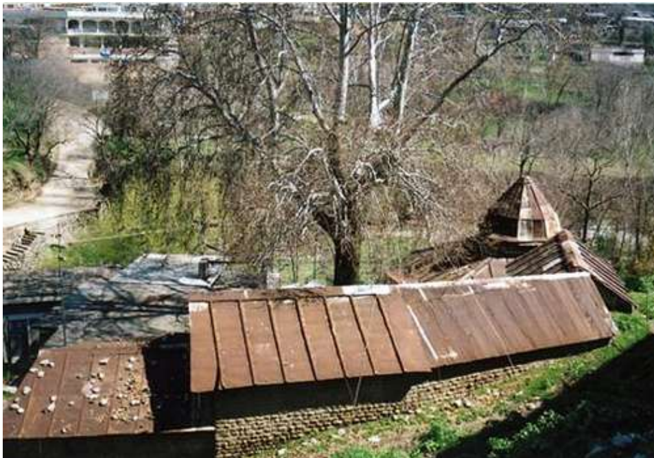
RECENT VIEW OF THE SHIV TEMPLE, PRIOR TO DAMAGE (COURTESY OF THE SHIV TEMPLE SOCIETY)
